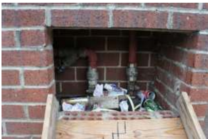
Example of building entry with uninsulated pipes at The Avenues
