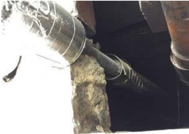
Example of connection to existing pipework from boiler house
